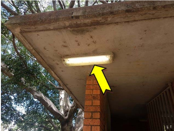
Photo 1. Exterior, throughout, single tube fluorescent light fitting – suspected PCB-containing capacitor.
